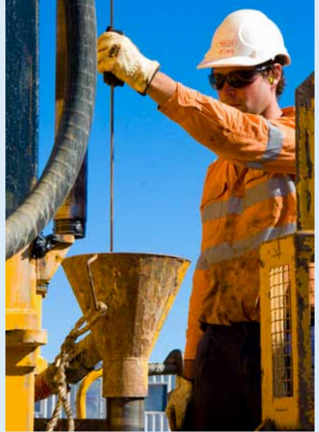
Injection testing solutions AGR Field Operations - Alternative Energy
